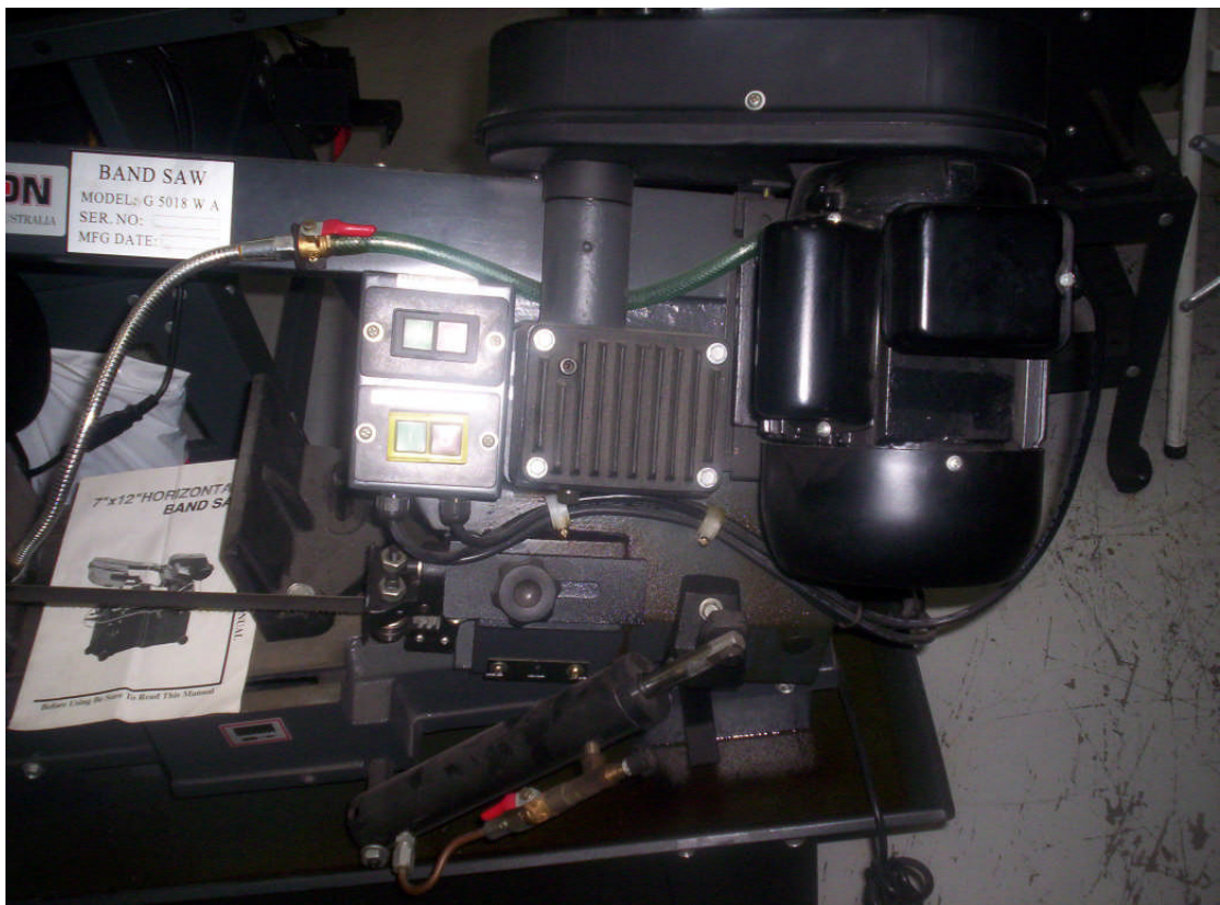
BAND SAW, the run and start capacitors are housed left on the side of the motor.
