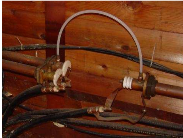
Figure 14.52: Flexible coaxial cables connected to rigid lines.
