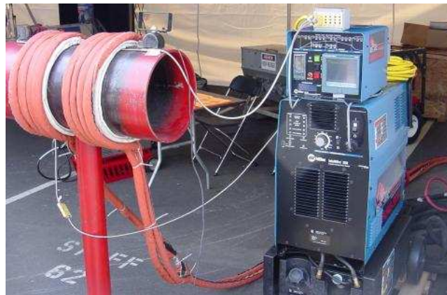
Figure 9.62: Induction heating: Primary insulated winding induces current into lossy iron pipe (secondary).
